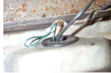
Note the green ground wire attachment as well as the correct installation on the wire grommet in the outermost light.
